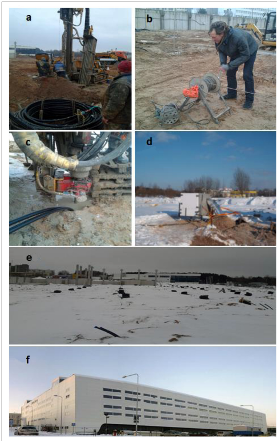
Fig. 2. Initial phase of the project: a – drilling the bore-hole; b – performing gamma log; c – installing the BHE; d – performing a TRT test; e – BHE field; f – completed building
