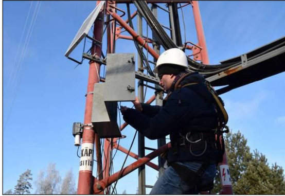
Fig. 9. The installation of the LOGGER NRG Symphonie PLUS3, hygrometer and a photovoltaic panel on the mast
