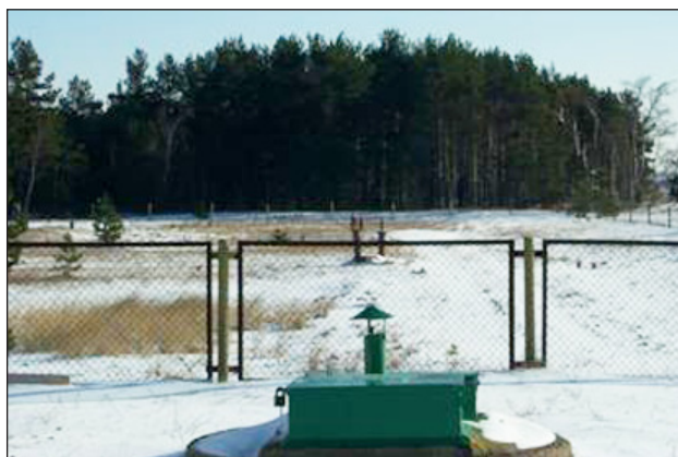
Fig. 1. Groundwater field with the top cover of borehole
